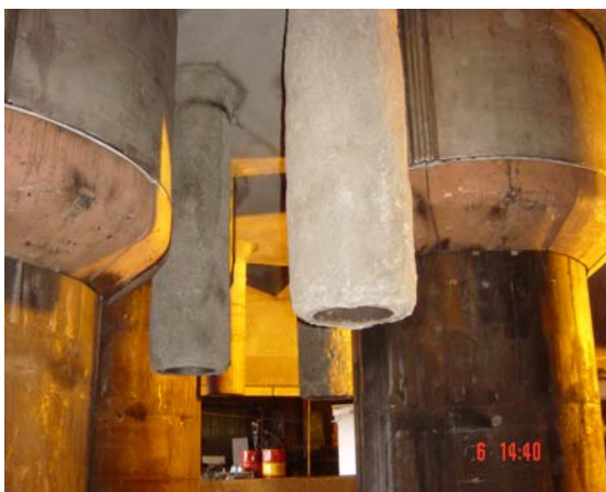
Figure 1: Current furnace electrodes
